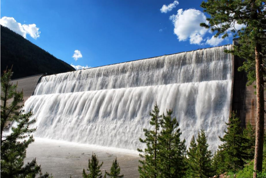
Figure 81. Water from the spillway of Upper Stillwater Dam flows from the reservoir and into Rock Creek, 31 miles northwest of Duchesne, Utah. (Reclamation photo.)
