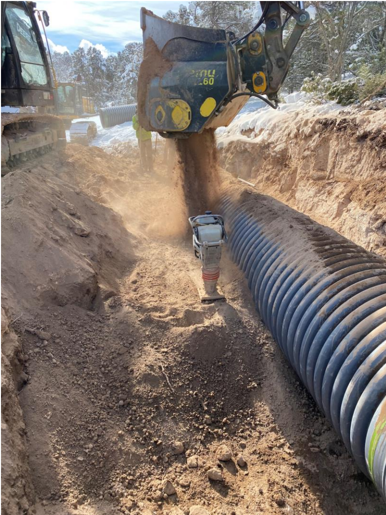
Figure 12. Backfilling Pipeline on Section Two of the Gould Canal Improvement Project B - in Crawford, Colorado
