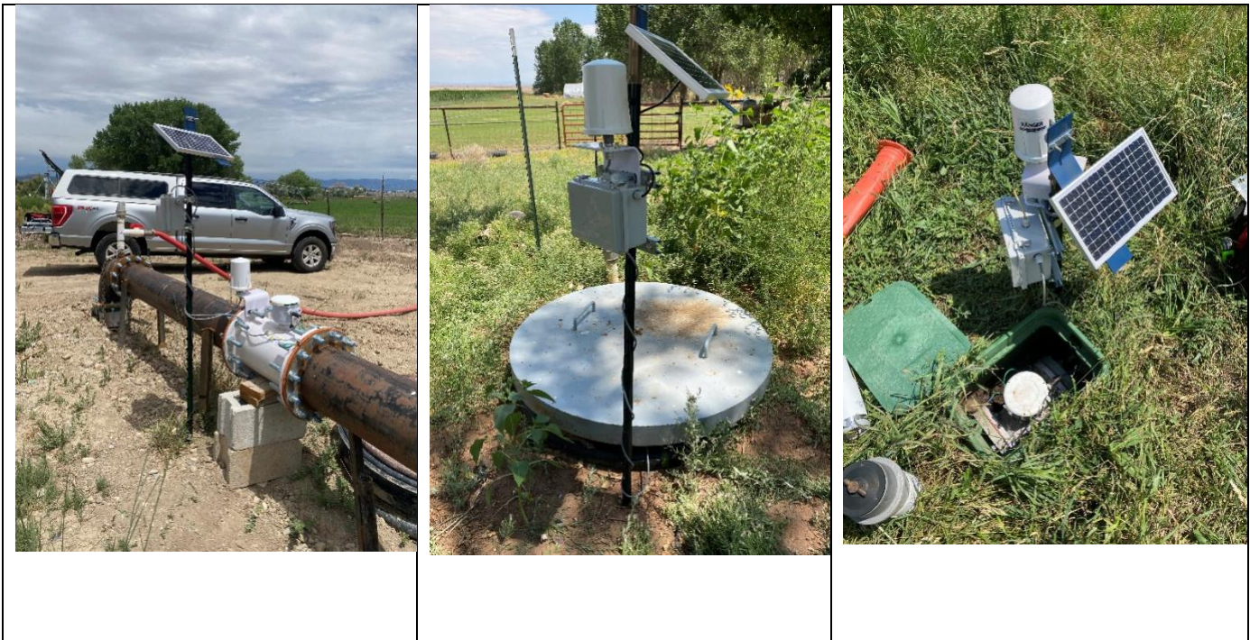
Figure 15. Flow meter installation with SignalFire Ranger telemetry inset
